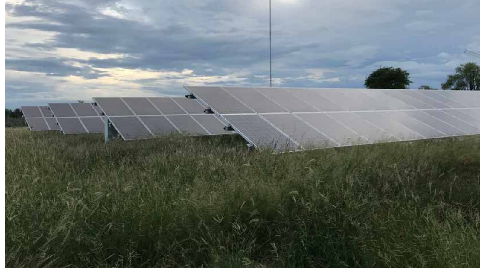
Tsumkwe Solar PV/Diesel Hybrid Mini-Grid System (303 kW) in Otjozondjupa, Namibia
